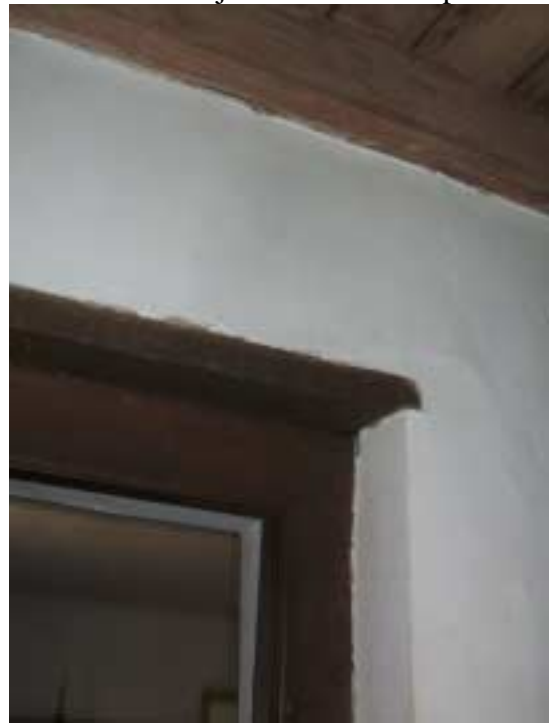
Interior door between units "A" and "B" recessed in the wall, 4" to the west.
