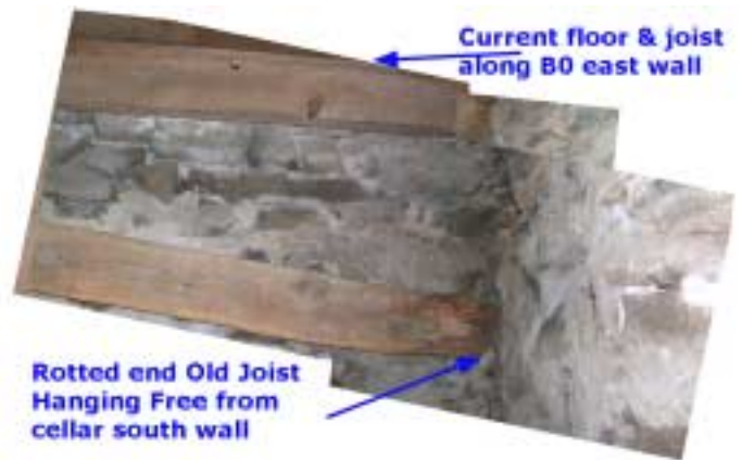
Close-up of rotted south end of old floor joist now disconnected from south "B0" cellar foundation and dangling free.
