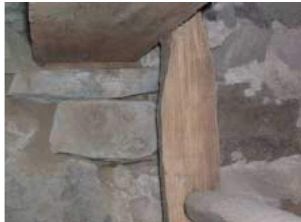
West end of summer beam rests on loosely piled rocks filling the pocket to bring the beam from its original position when unit "A" & this wall were built to its new position when hearth extension built..
