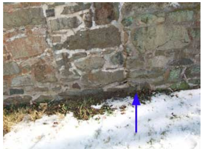
North wall Vertical seam jogs 4" to the east from unit "A", resulting in a ground-level notch
