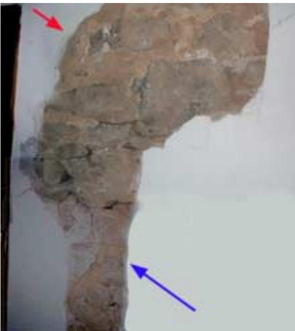
Red Arrow shows mortar with exterior finish. Blue arrow shows rough, unfinished interior garret mortar. Pencil diagonal line drawn on plaster shows the conjectured south roof slope, based on mortar.
