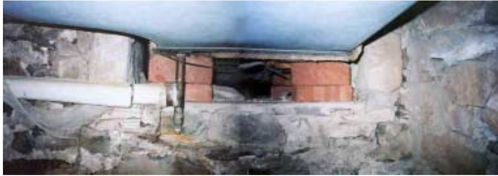
Opening in north wall "B0" to shed crawl space. HSR says wood sill [at base of opening] may date to an older structure. Brumbaugh says same for lintel (obscured by ductwork). West face Fireplace mass to right.
