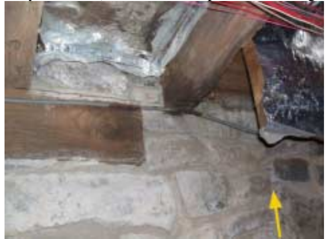
Summer beam embedded in west facing hearth extension (everything to left of yellow arrow) indicating floor was raised to new level when hearth extension added.
