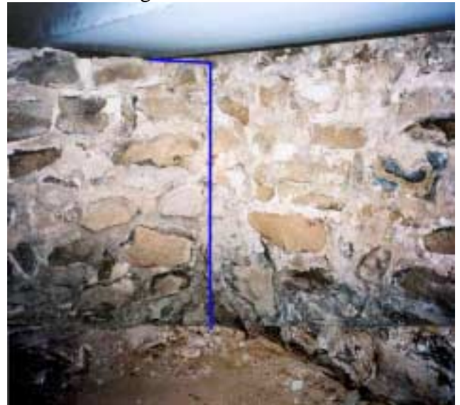
Blue line shows top and north end of west wall as it abuts north wall. North wall existed when west wall built.
