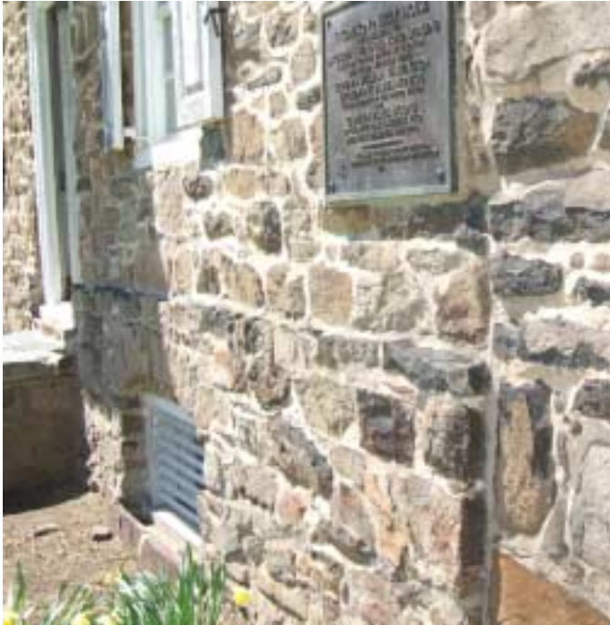
South exterior of unit "A". water table protrudes horizontally midway between cellar and 1 st floor windows. It is noticeable in jagged shadow and shadowed edge at "A" – "B" vertical mortar seam
