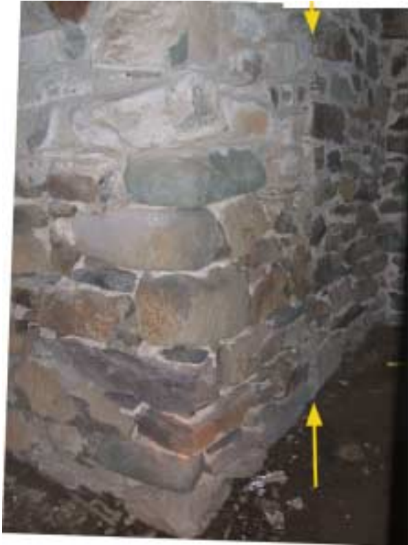
S-W "B0" corner fireplace mass- primarily hearth extension underpinning. Stones nearer floor are smaller. Yellow arrow indicates vertical groove delineating extension from original mass. East cellar wall in background.
