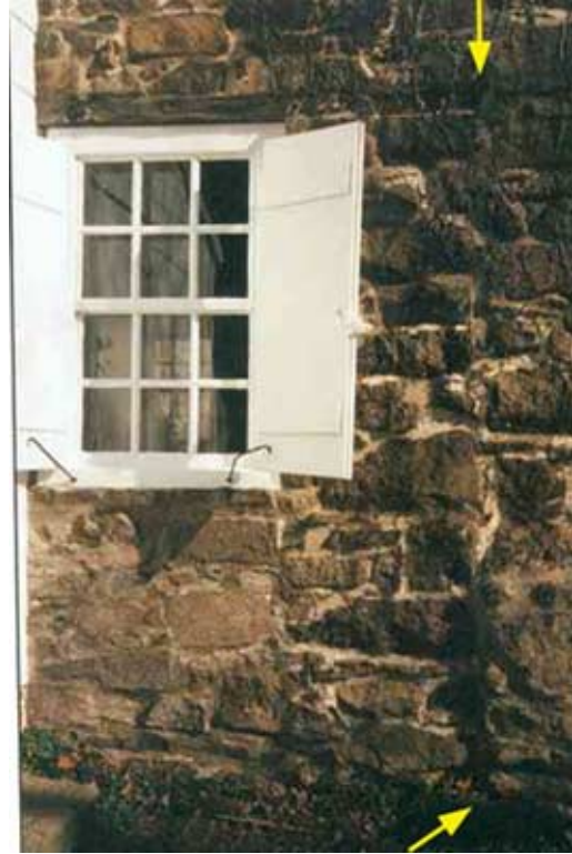
Unit “B” north exterior shows where a doorway has been filled in to hold a window. Yellow arrows indicate vertical seam with unit “A”. Note wooden “plate” over window. Lower arrow indicates location of ground-level 4” jog to the east of vertical seam.
