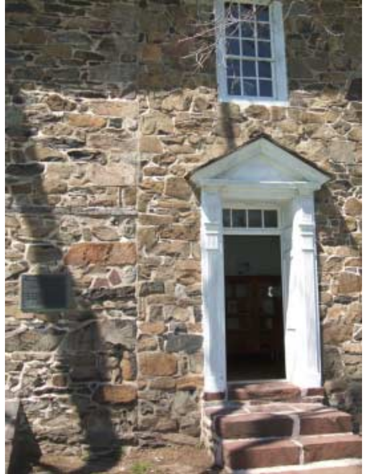
Vertical seam separating unit "B" from "C" on the right. Note large stone quoins forming SE but not SW corner of unit "B".
