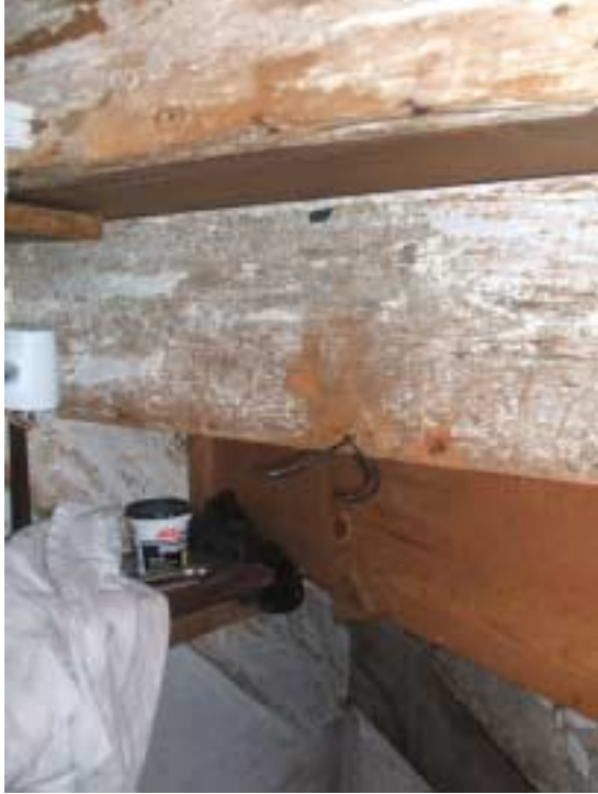
White-washed underside of stairs between 1 st & 2 nd floors of unit “B”, indicating there once was a parallel set of stairs underneath them leading to the south-east cellar of “B0”.
