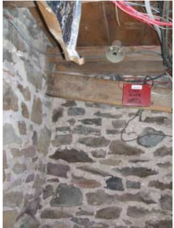
Current floor joist above old, sagging floor joist along east end of "B0" cellar. North end of old joist embedded in "B0" fireplace mound.
