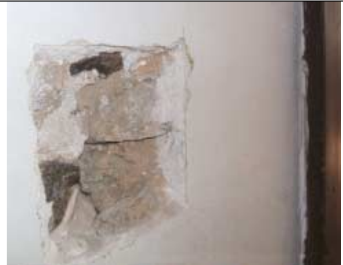
Removal of plaster to take mortar sample M13 from south side of south jamb of unit "B" fireplace reveals fireplace construction. Door from "B" to "C" visible to right.
